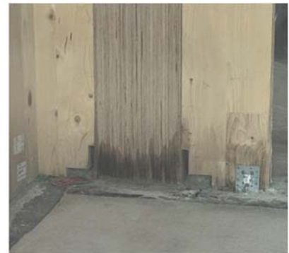
Figure 1. Detail on site of observed moisture uptake of a column made of beech LVL (photo taken in February 2024).
